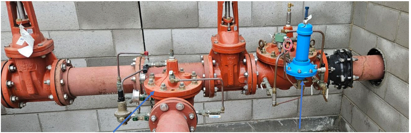
4" Pressure Reducing Valve (PRV)
