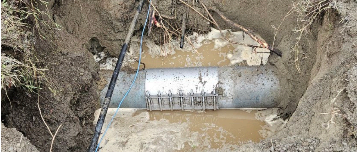
10" Patch requiring correction
