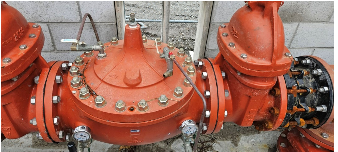
10" PRV opens for very high-water demand conditions (allowing full flow from HBMWD)
