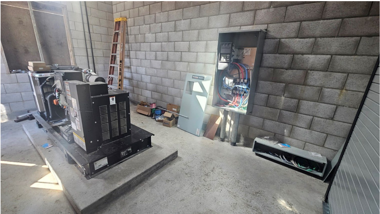
New 75KW Generator
