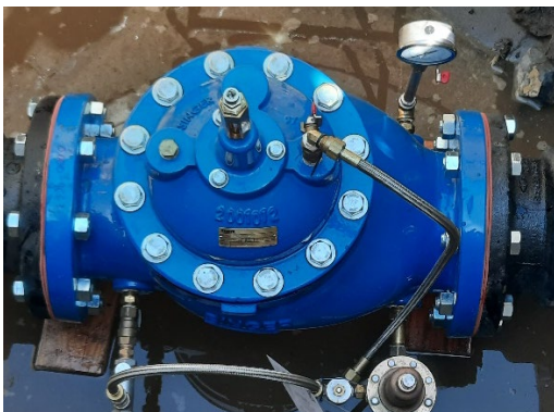
6" PRV Feeding system directly from HBMWD
