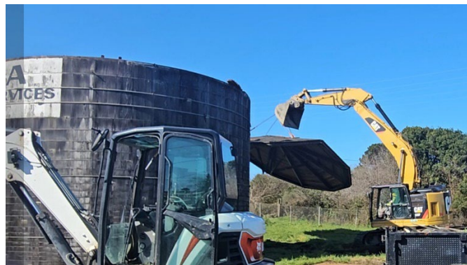
100,000g Redwood Storage Tank Decapitated
